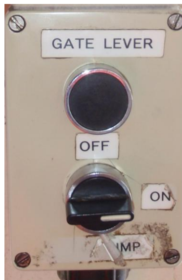
Photograph 5 – Gate Lever Lock
