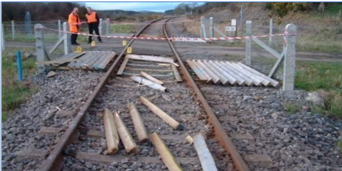
Photo 1 - Damage to infrastructure
