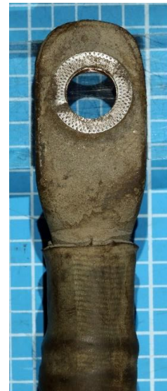
Figure 17 – S1 Earth Shunt Cable Lug furthest from the failure
