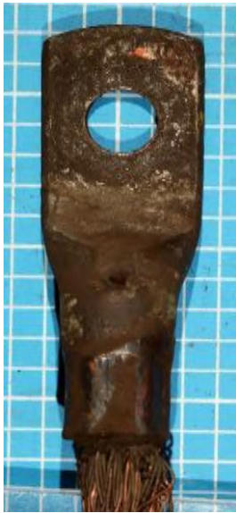
Figure 15 – S1 Current Return Cable Lug closest to the failure
