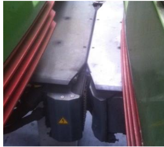
Figure 10 – Closed electrical head cover
