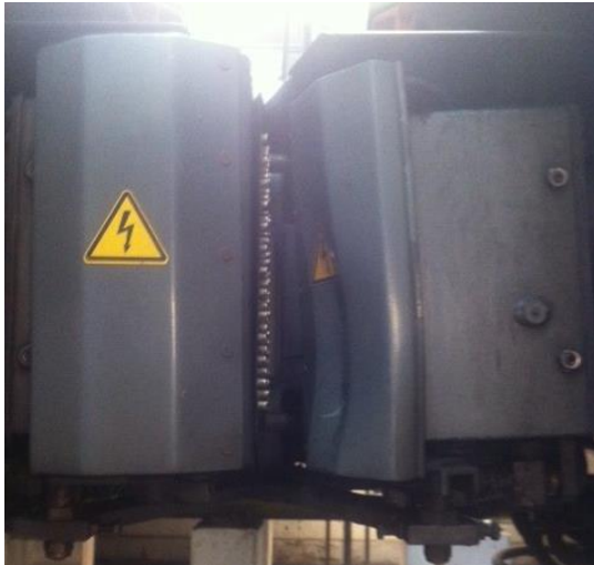
Figure 9 – Damage to electrical head cover
