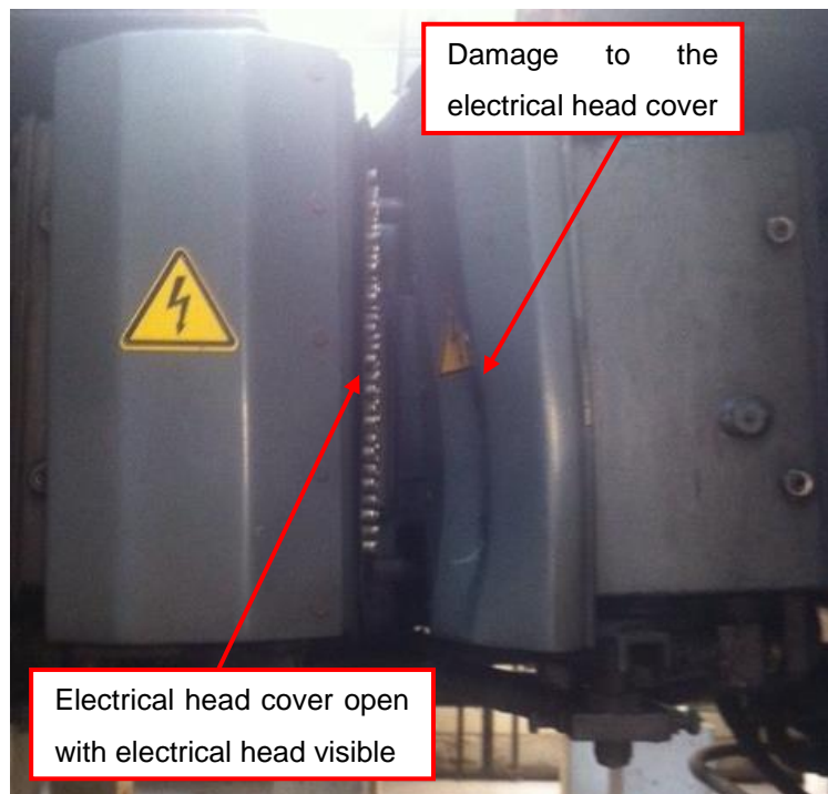
Figure 3 – Damage to coupler electrical head cover
