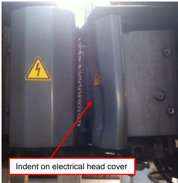
Figure 12 – Indentation on electrical head cover
